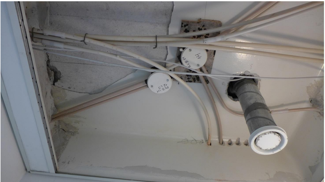
An original ceiling fragment in one of the 4th floor toilets, above the dropped ceiling structure hiding the 1970's and later HVAC-installations. The gloss of this fragment is not as distinctive as it probably has been in more important spaces like entrance hall or lounge in the first floor.
