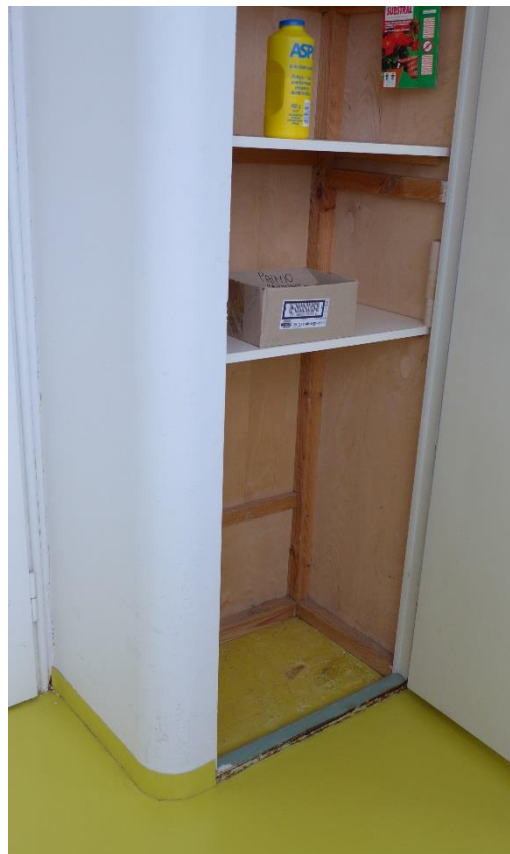
The original fragment of yellow flooring in comparison to the renewed flooring surrounding the cupboard.
