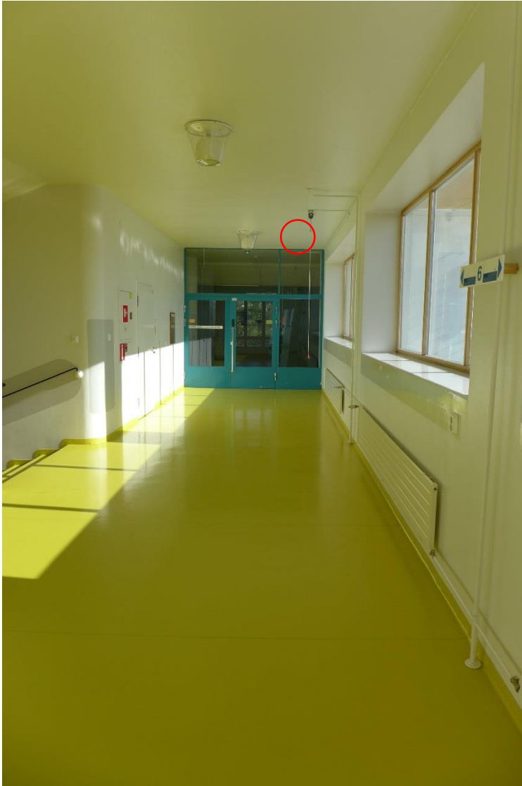
The fifth floor main staircase. The spot where cross section sample was taken.
