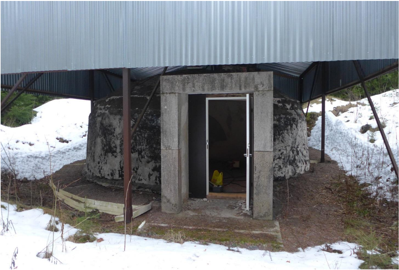
The state of Rose cellar today. The masses of soil covering the dome have been removed. The original moisture insulation, the black tar-like coating has been scraped down to ensure further drying of the structure. The cellar has been covered with a temporary shelter to protect it from rain and subzero temperatures during 2005. The original door has been removed, stored and replaced by a temporary door. An underground drain has been installed around the dome to gather most of the water from the ground.
