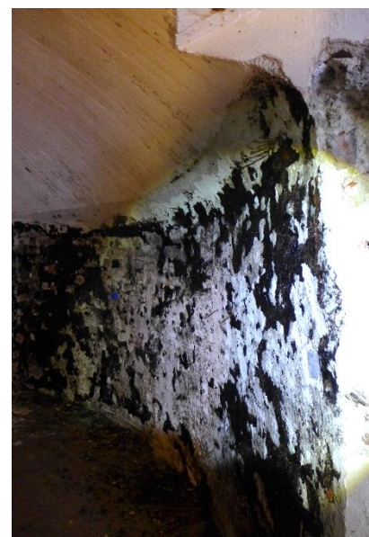
The state of the walls inside the cellar. Tar-like coating has been partly stripped to help the drying process of the structure.
