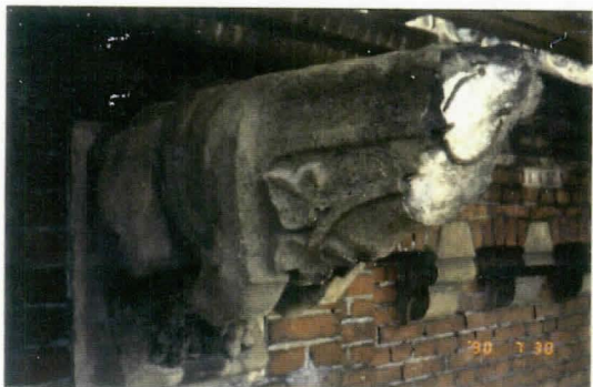
UNTIL ONE OF THE HEADS WAS DIS-LODGED BY A SLIGHT BUMP! A RUSTED IRON RING HAD CAUSED CRACKING. THE DEEP CARBONATION CAN BE OBSERVED.
