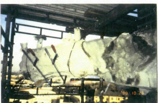
CASTING THE HEAD PART TO ONE OF THE UPPER GARGOYLES. THE MOULD IS SUPPORTED WITH A GLASS-FIBRE CASE AND SECURED WITH IRON BANDS AND SCREW CLAMPS.
