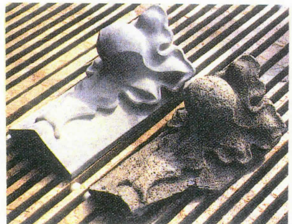
A NEW CROCKET AND A DETERIORATED ONE
