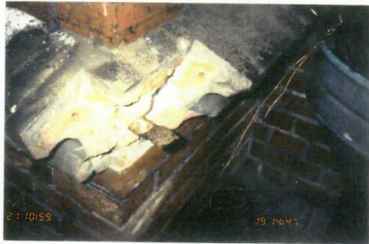
A RUSTED PIECE OF REINFORCING IRON HAS BROKEN THE CORNER OF A MOULDING. THE CORNER HAS BEEN CUT OFF.
