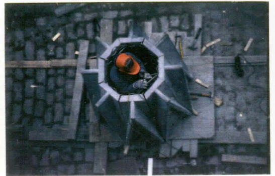
ASSEMBLING THE PRE-CAST UNITS OF THE CORNER PINNACLES OF THE TRANSEPTS TO BE LIFTED UP.
