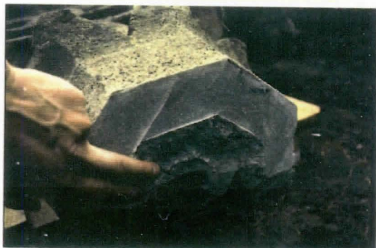
THE CENTRAL STEEL BAR AND THE CAST CEMENT MATERIAL OF THE LOWER PART WERE IN PERFECT CONDITION.
