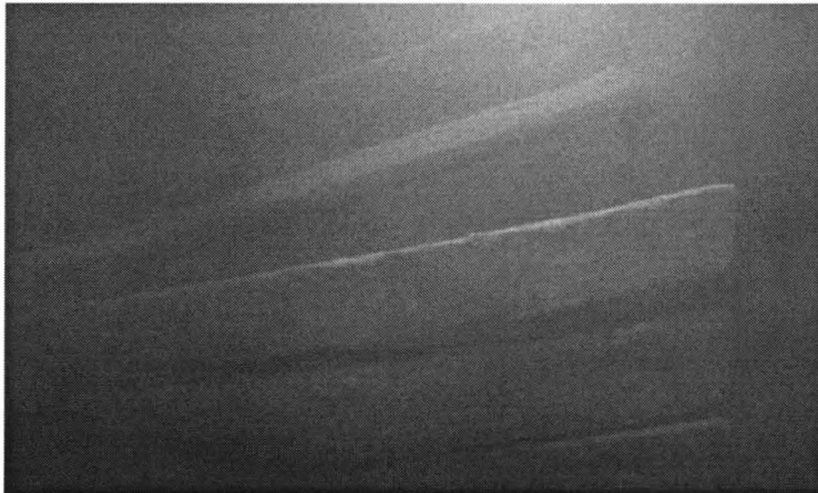
Picture 47. The main wale on both sides has become loose from the stempost. Picture taken from the starboard side. Photo by P. Raasakka & J. Kaasinen.
